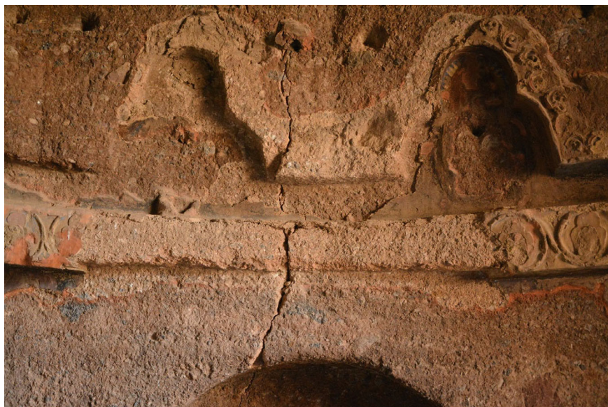
Fig. 2 Detail of Cave D frame, at the base of the dome. Fractures cross the stone walls and the painted plasters, causing their detachment and loss
